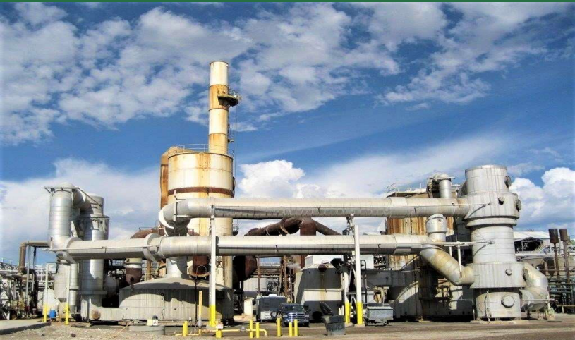
Sulfuric acid plant
